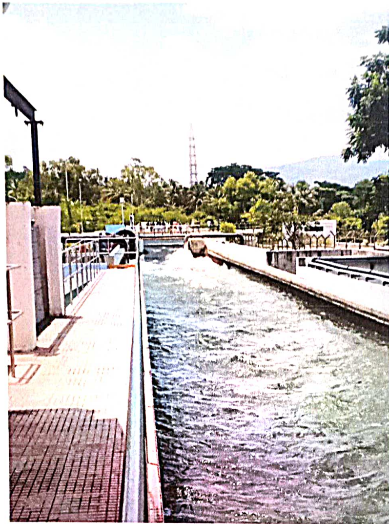
Water comes from aerator to tanks
